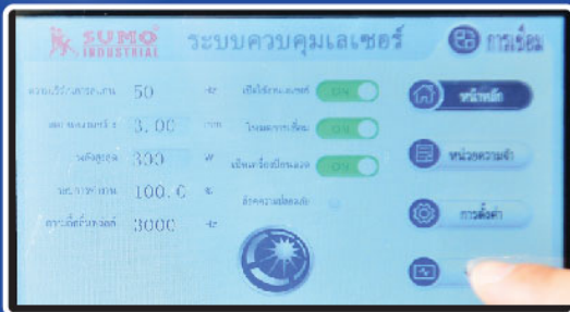
Control system brand SUMO INDUSTRIAL
